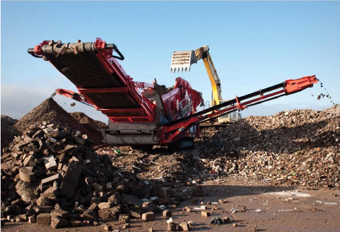
Figure 3.2-3: Example of Mobile Screening Plant
