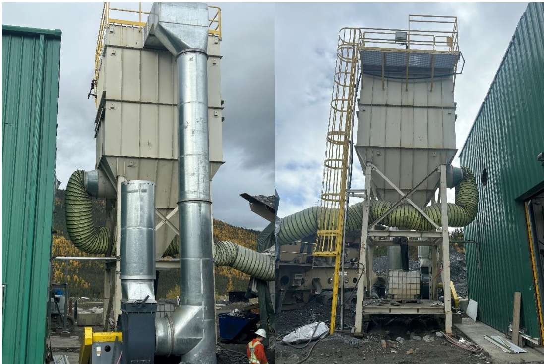
Figure 5-1: Dust Collection and Ventilation System
