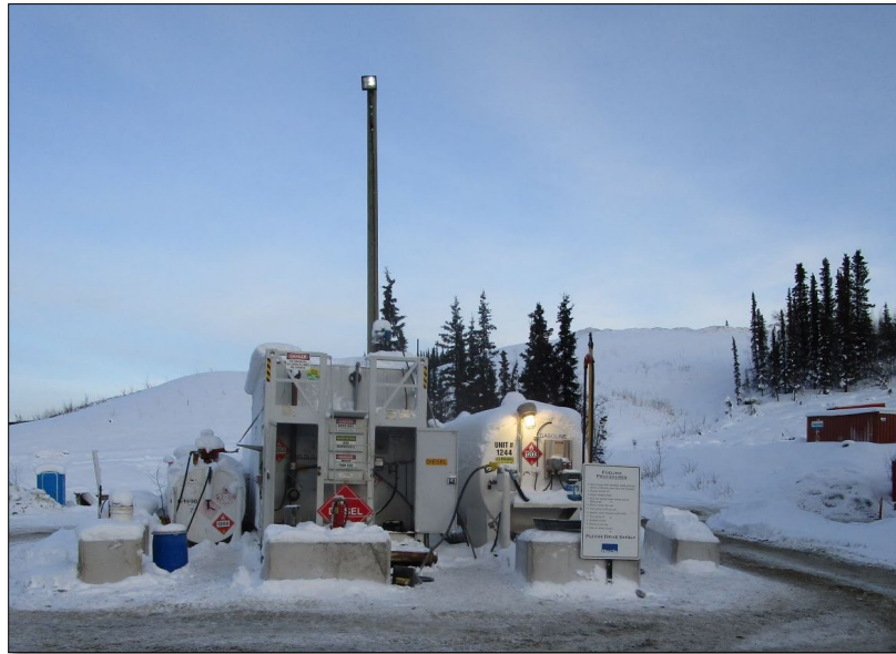
Photo 3-9: Diesel and Gasoline Fuel Tanks
