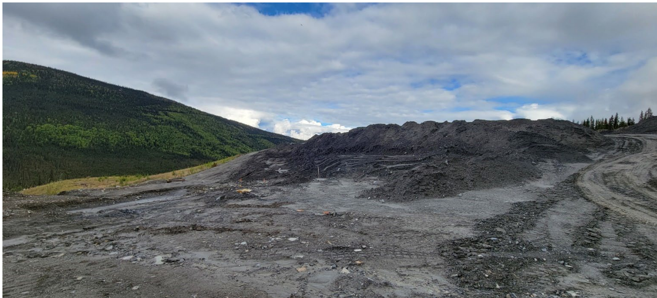
Photo 14: DSTF Phase 1A area, near top, south end. Loose, poorly graded, and uncompacted tailings visible. VDS visible in left of frame. Facing north. (I. MacIntyre, Aug. 28, 2022)
