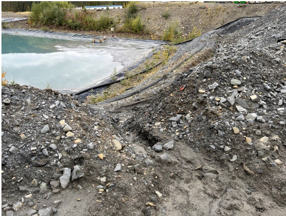
Photo 13: Mill water storage ponds, erosion gully – facing east (R. Trimble, Aug. 28, 2022)
