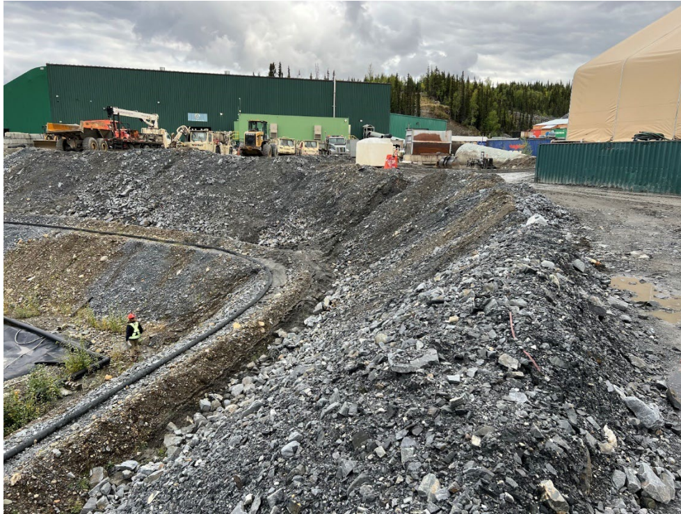
Photo 12: Mill water storage ponds, erosion gully – facing northeast (R. Trimble, Aug. 28, 2022)
