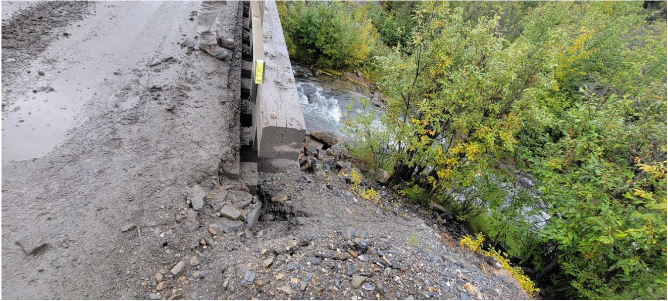
Photo 7: Lightning Creek Bridge - Bellekeno Haul Road, erosion gully forming along road edge (I. MacIntyre, Aug. 28, 2022)
