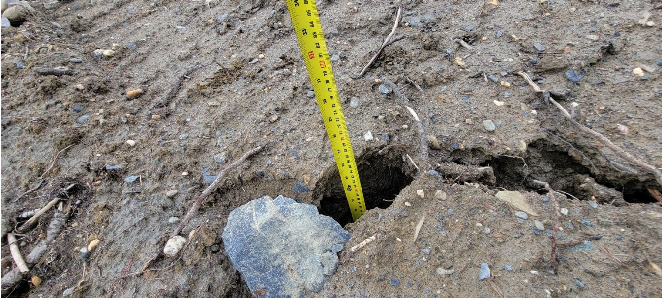
Photo 16: DSTF Phase 1A area, near top, north end. Sloughing of loose, uncompacted cover material. Crack approx. 60 cm deep. (I. MacIntyre, Aug. 28, 2022)
