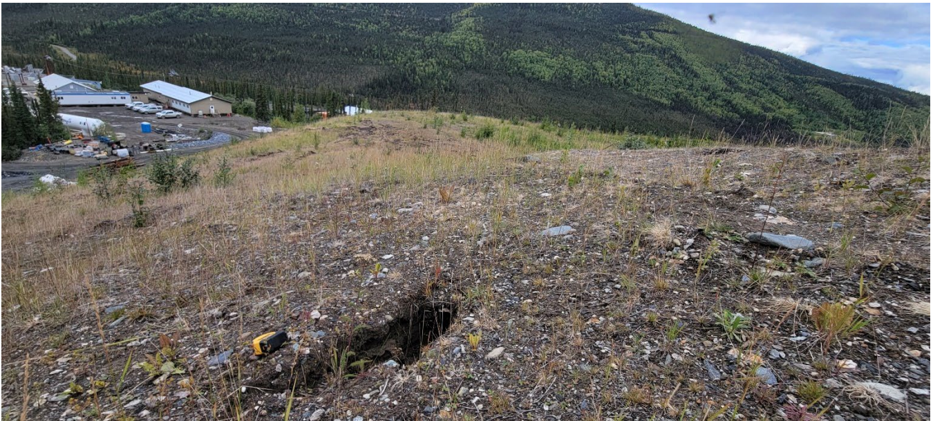
Photo 17: DSTF Phase 1A area, southwest slope. Small sink hole indicating migration of materials. Appears to be limited mostly to cover material. Facing west. (I. MacIntyre, Aug. 28, 2022)
