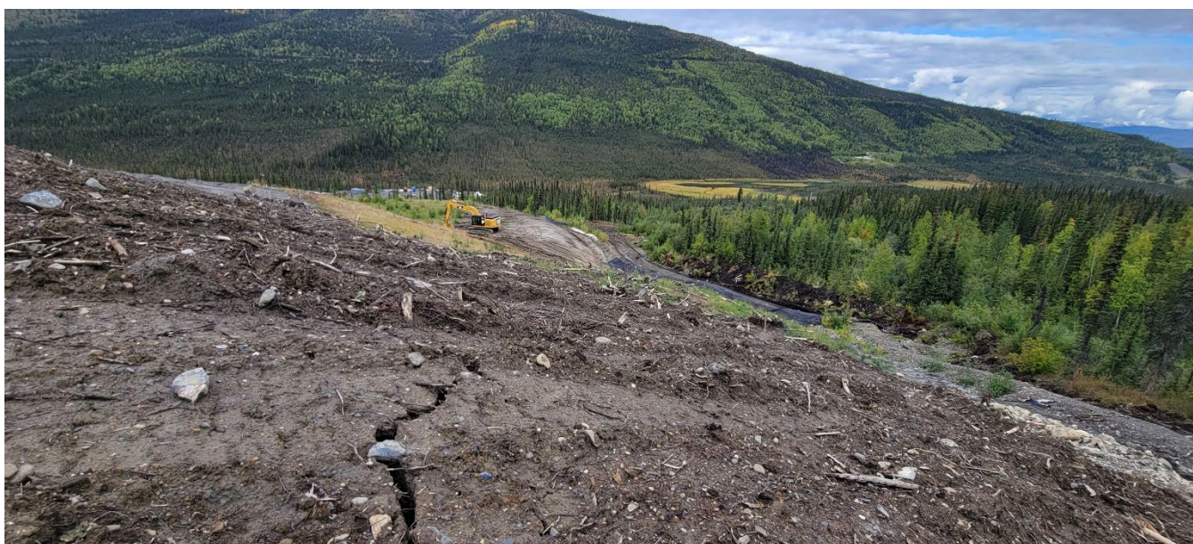
Photo 15: DSTF Phase 1A area, near top, north end. Sloughing and cracking of loose, uncompacted cover material. Facing west. (I. MacIntyre, Aug. 28, 2022)
