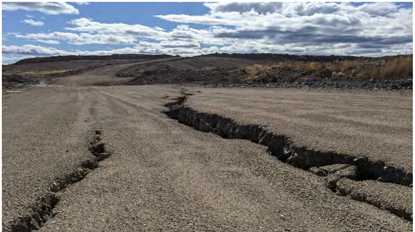
Photo 6-4: Longitudinal cracking along the crest of the SWD first observed in 2019..
