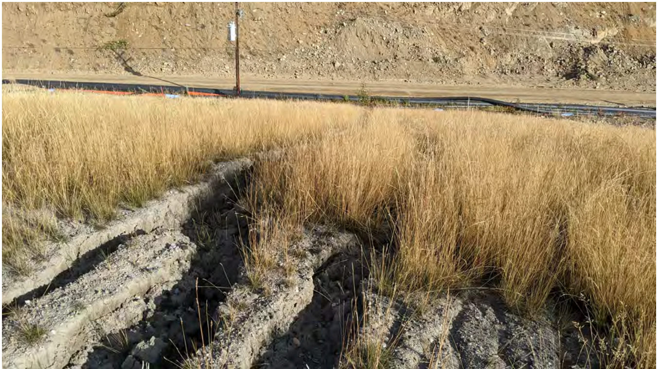
Photo 2-4: Erosion gullies, looking north towards the main access road.
