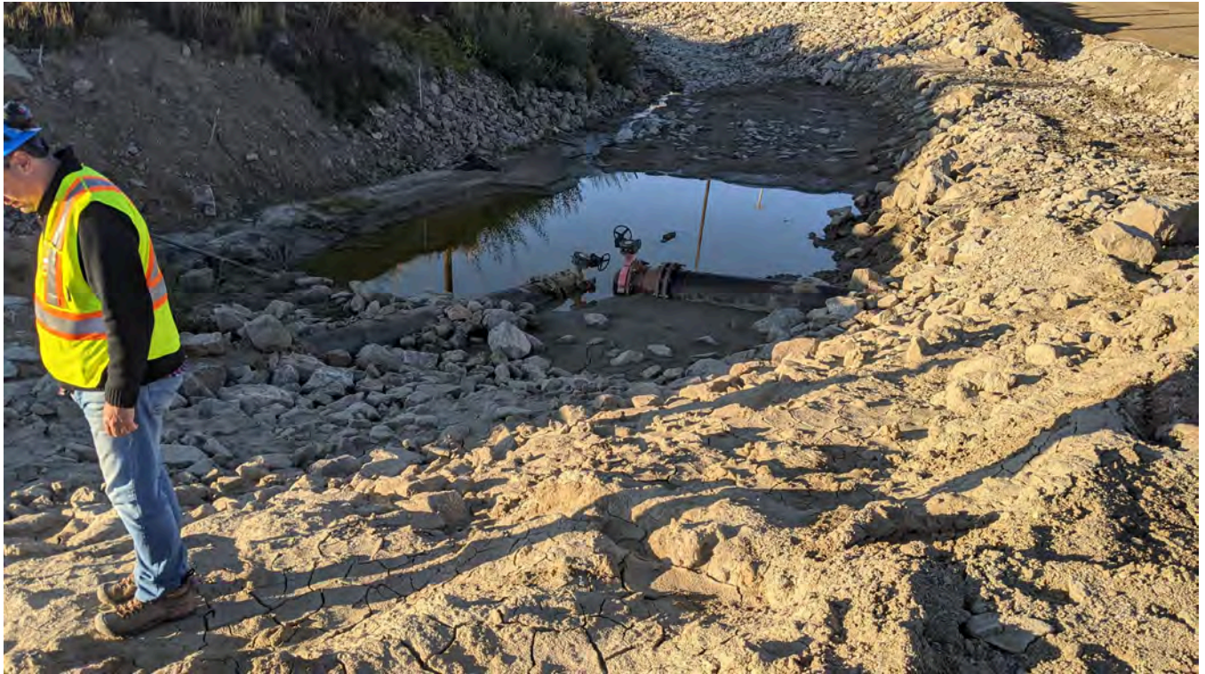
Photo 3-1: TDD Intake Channel. Photo taken from the Airport Access Road looking upstream. Grading of the Underground Access Road results in surface runoff being directed into TDD intake. The intake area was cleaned-out prior to the inspection.
