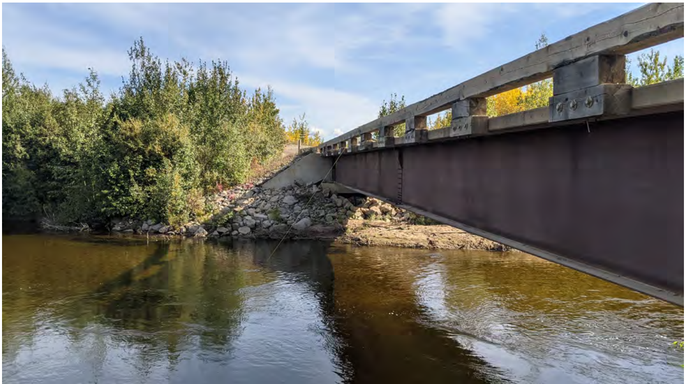
Photo 13-4: Downstream end of the eastern abutment. A rope is suspended from the bridge by the Minto Environmental department for environmental monitoring of the creek.
