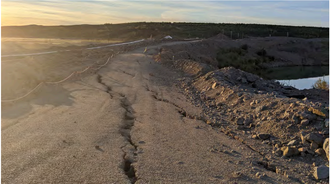
Photo 15-3: Cracking along inactive access road along pit rim.
