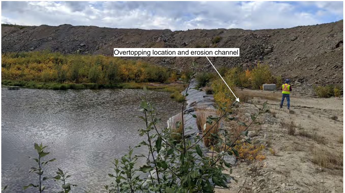
Photo 14-9: W15 Sump south of the Main Pit. The sump appears to have overtopped in the past year with water infiltrating through a sinkhole into the pit.
