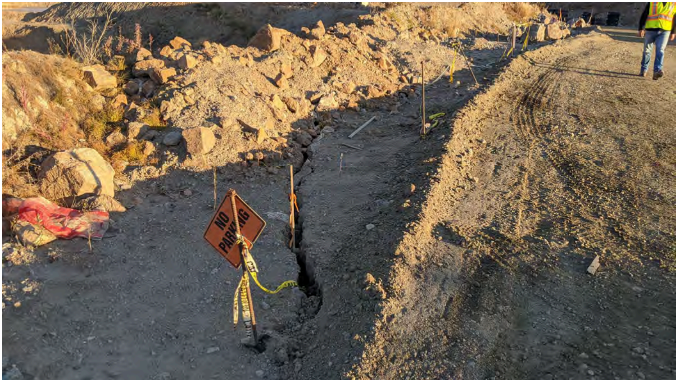
Photo 15-8: Cracking along the Area 2 Stage 3 Pit rim near the Underground Shop.
