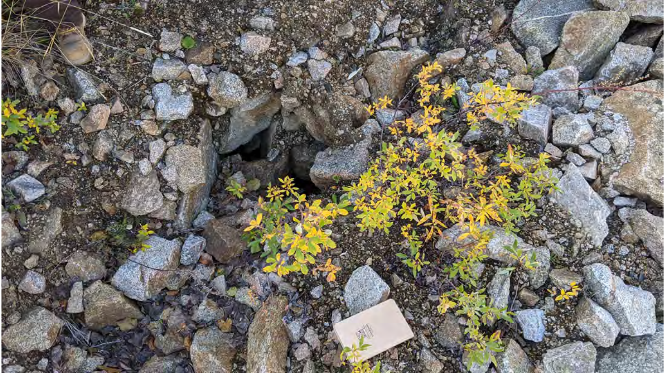
Photo 12-7: Potential minor sinkhole or burrow on the downstream south abutment near ground temperature cable WDT-08. No apparent change in condition since first observed in the 2019 inspection.
