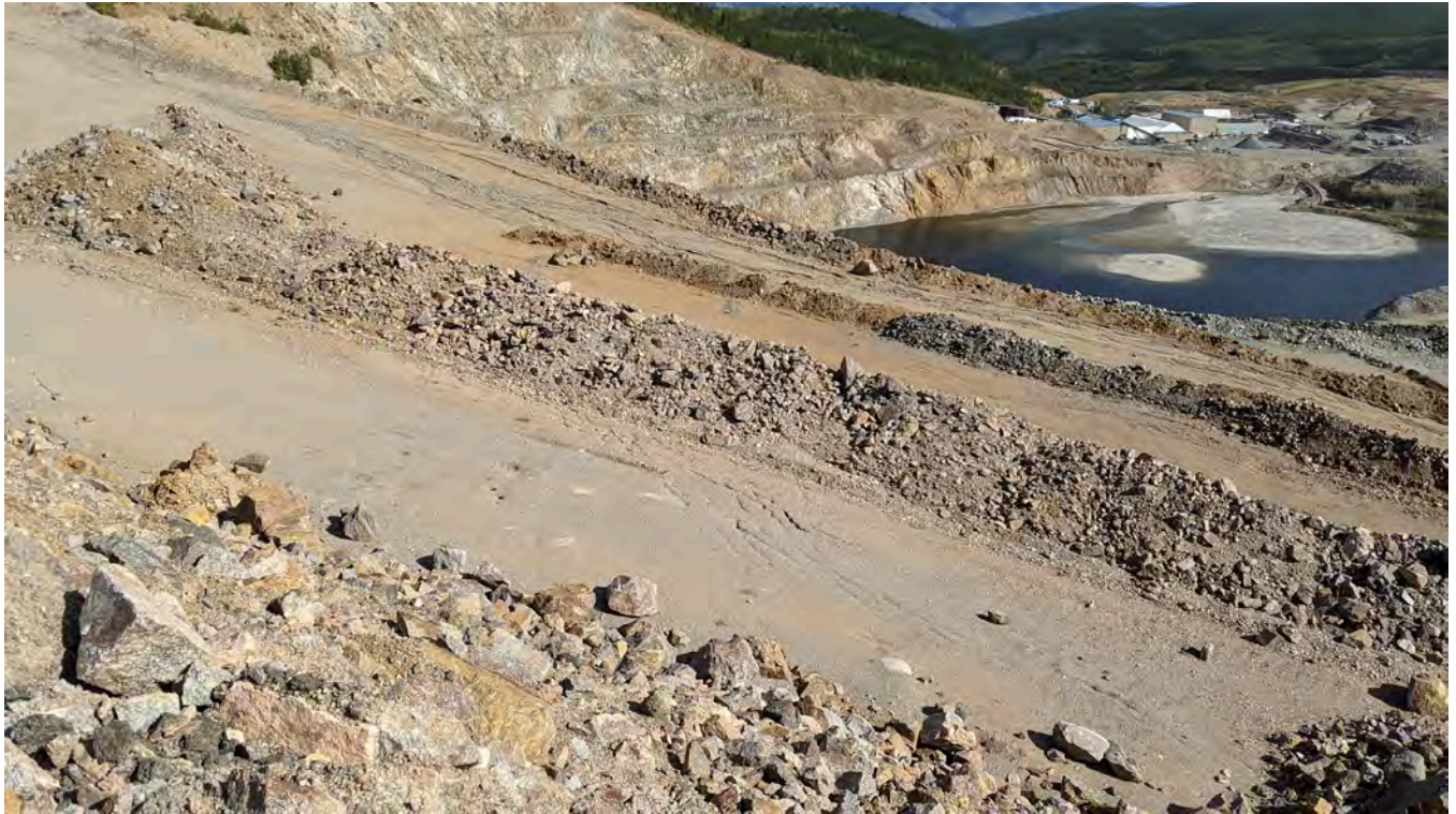
Photo 5-1: Cracking on the crest of the lower bench of the MWD Wrap.
