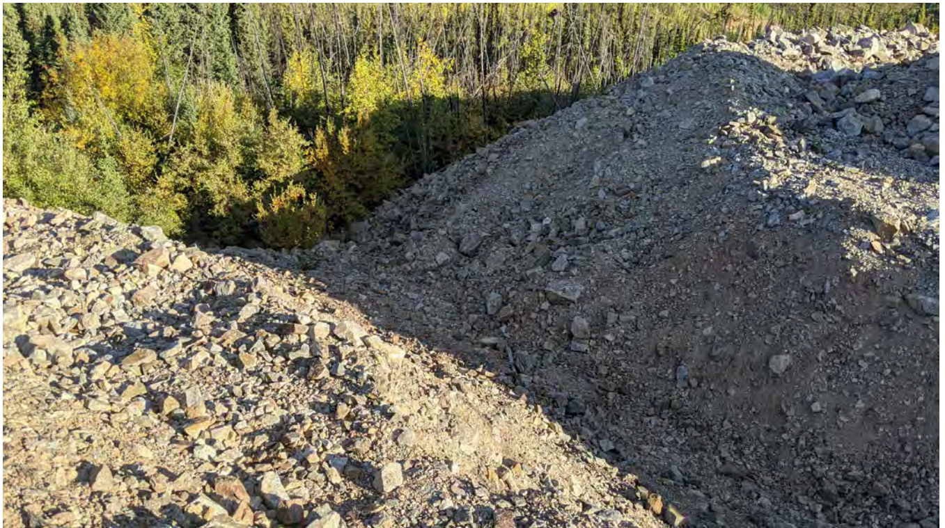
Photo 3-6: TDD Outlet. No flow was observed at the time of the inspection.
