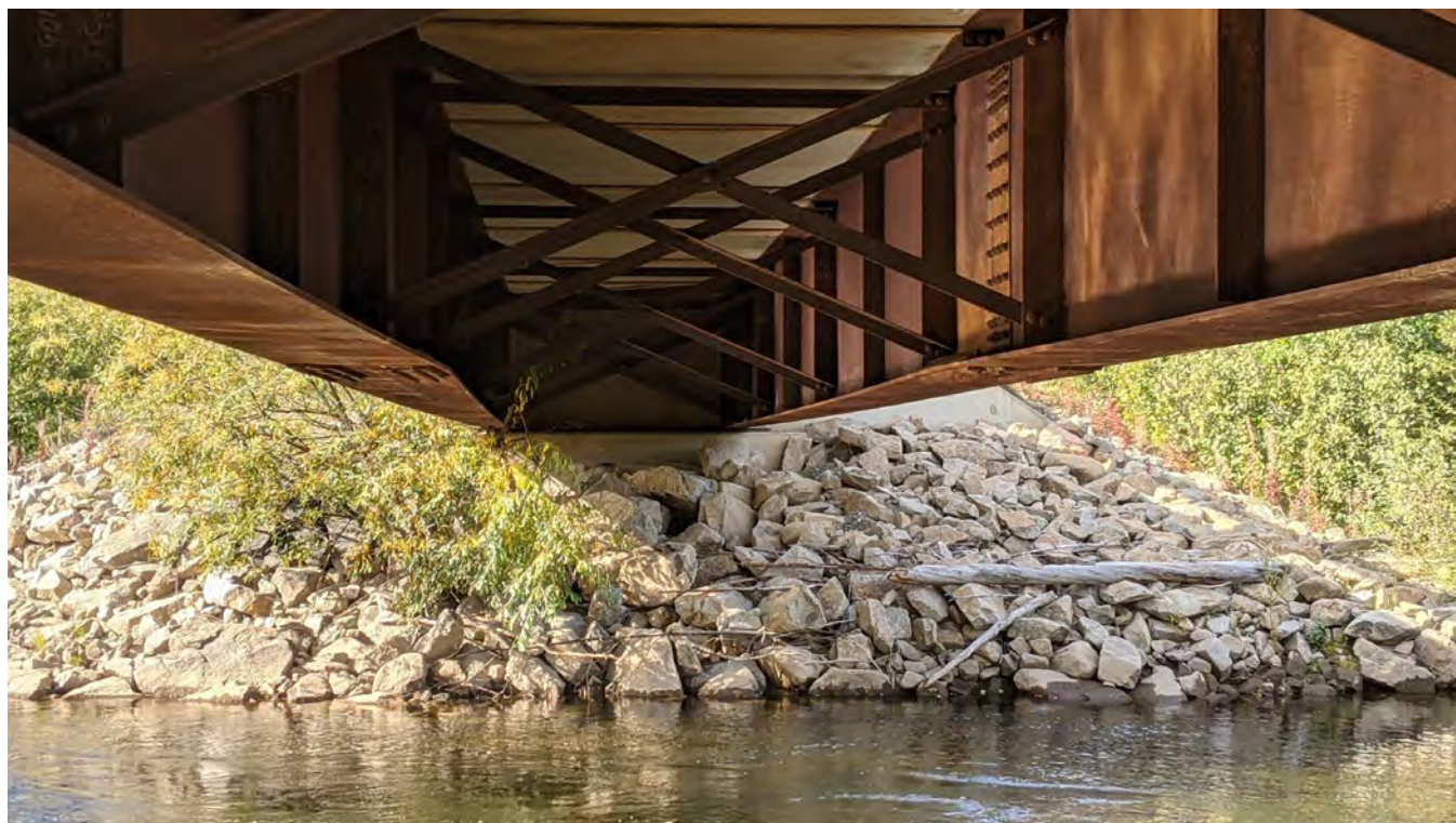
Photo 13-2: Western abutment. A Tree is growing on the upstream side of the western abutment.
