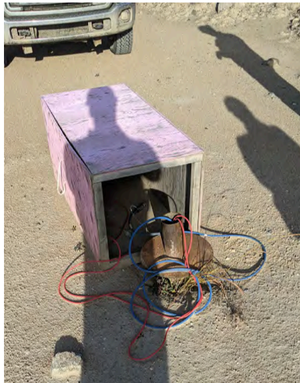
Photo 1-8: Piezometer DSP-06 and Thermistor DST-11 on the DSTSF waste rock crest. The instrumentation was found to be uncovered and exposed to the elements. Precipitation down the borehole could influence the instrumentation readings.
