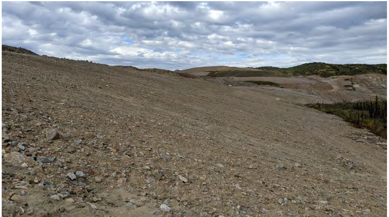
Photo 6-6: Reggraded SWD slope below the longitudinal cracks.
