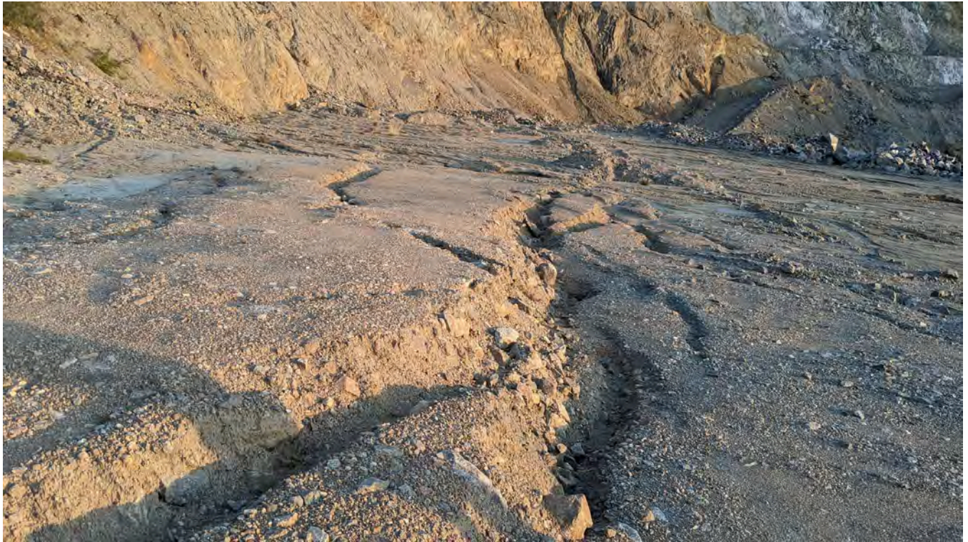
Photo 14-8: Historical cracking of the In-Pit Dump above the SAT Dump. The cracks are filling-in and near-by survey hubs indicate no current movement.
