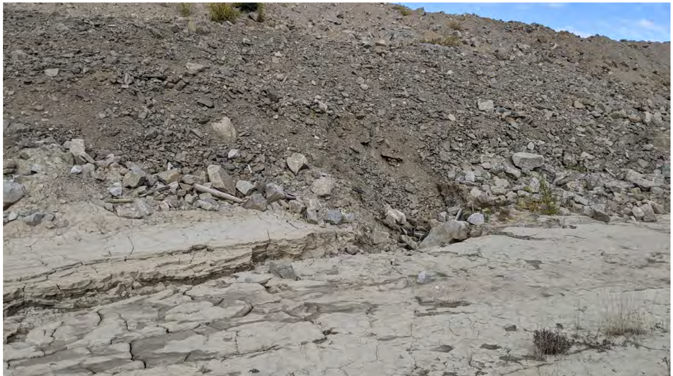
Photo 14-10: Lower end of the erosion channel and sinkhole beneath the haul road..
