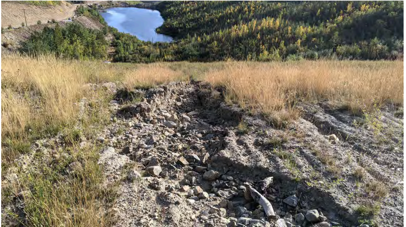
Photo 2-3: Erosion gullies – looking east towards the WSP.
