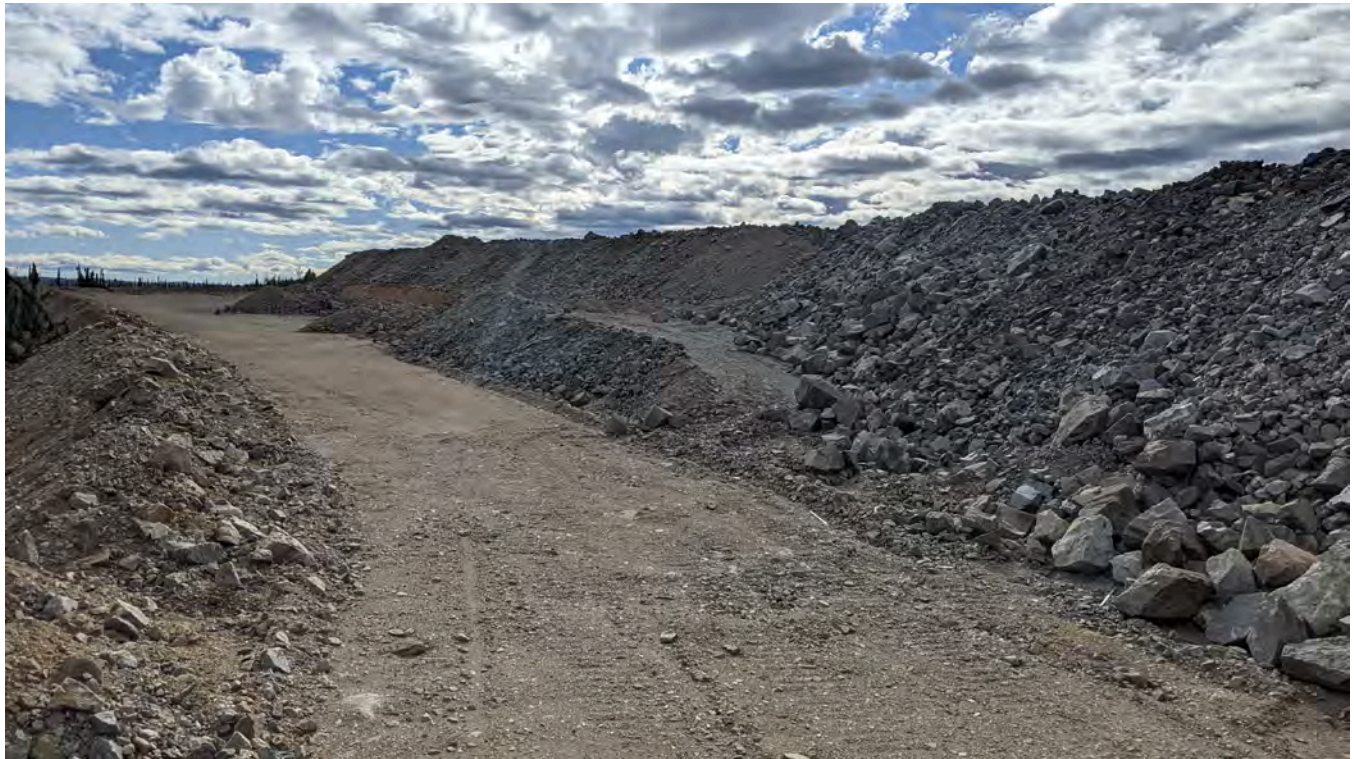
Photo 6-5: HGW Pad at the south end of the SWD
