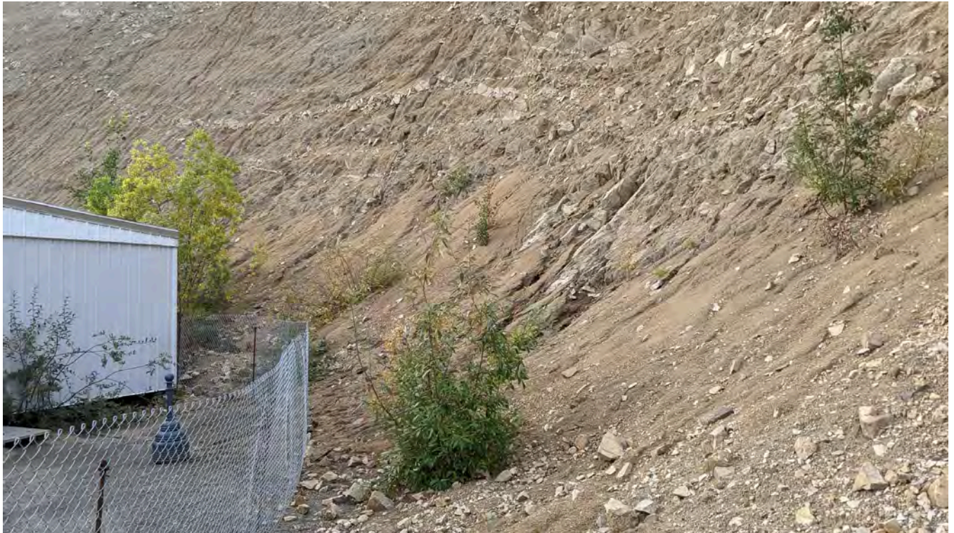
Photo 9-3: Historical seepage location located at the northeast corner of the mill area. No seepage was observed at the time of the inspection.
