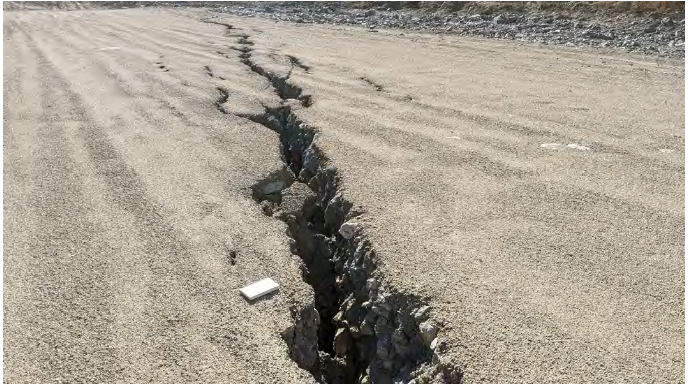
Photo 6-5: Longitudinal cracking along the crest of the SWD first observed in 2019 at its widest point.
