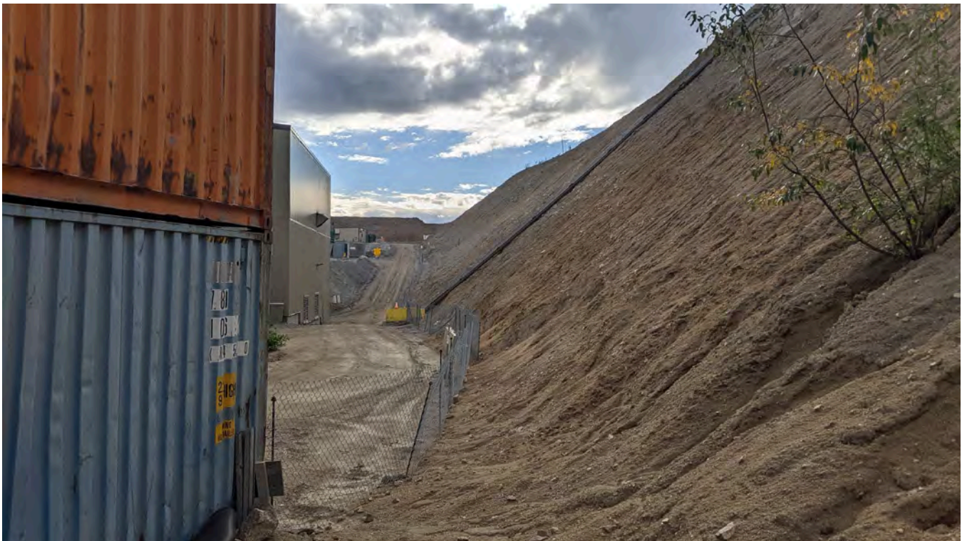
Photo 9-4: Minor slope erosion on the highwall.
