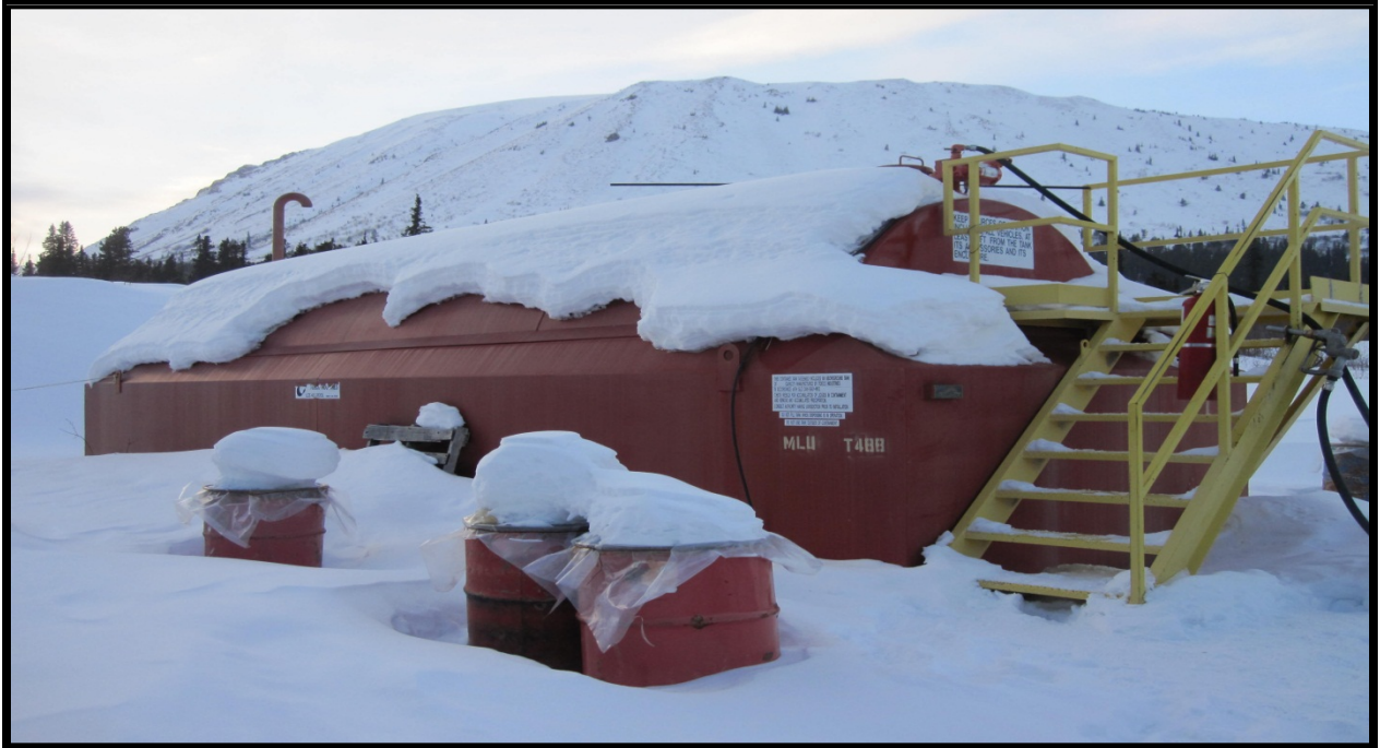
Photo 2-1: Main diesel storage tank, capacity 45,000 litres (photo taken March 19, 2011)
