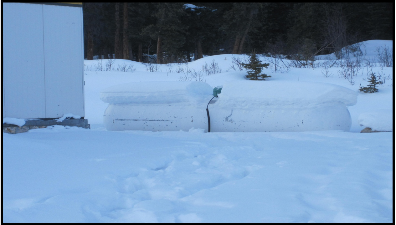
Photo 2-4: One of the five propane tanks (Table 6-1, photo taken March 19, 2011)
